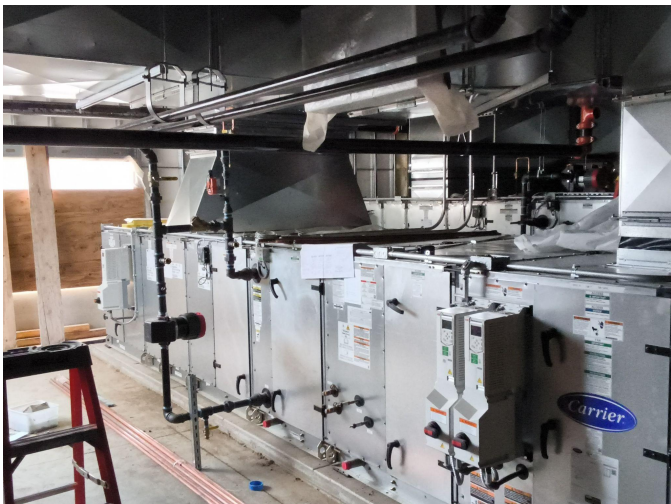
Air handling units
